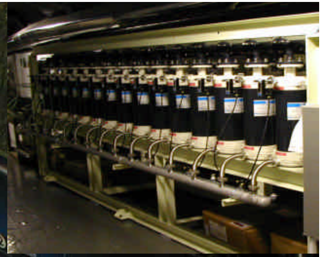
A bank of filters
